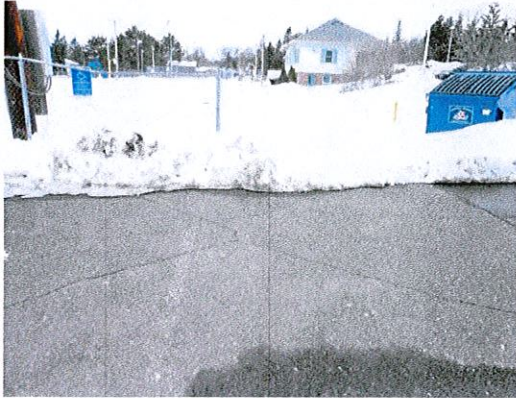
Photo 1: Re-stripe the accessible parking space (currently faded). Ensure the aisle aligns with the route the upper and lower levels.
