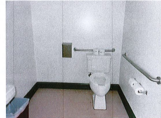
Photo 6: The upper level toilet rooms have been remodeled to provide features of accessibility. This is a good example of accessibility. Add a vertical grab bar and relocate the sanitary waste receptacle to below the side grab bar.
