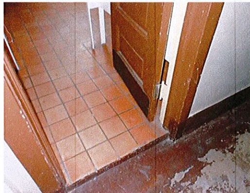
Photo 5: There is currently a 3" rise into the lower level toilet rooms. No features of accessibility are provided within the toilet rooms.
