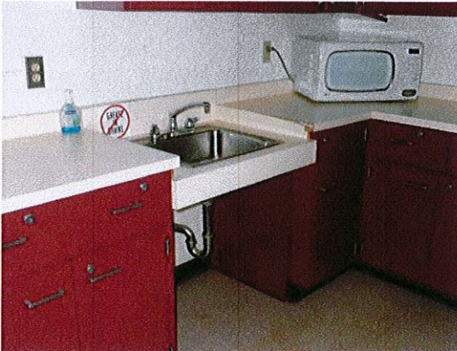
Photo 4: A sink with 26" (vs. 27" minimum) knee clearance is currently provided in the kitchen.
