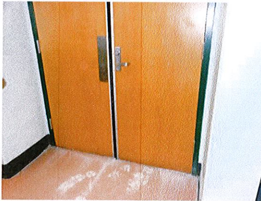
Photo 4: There are 3 sets of double doors leading into the gym. Modify 1 set so a single leaf provides a 32" clear opening.
