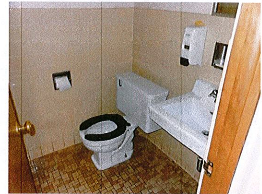
Photo 6: View of single user toilet room on main level. An accessible toilet room is not provided in the fire hall portion of the building.
