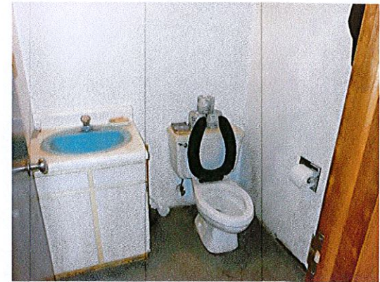
Photo 3: The single user toilet rooms do not currently provide any features of accessibility.
