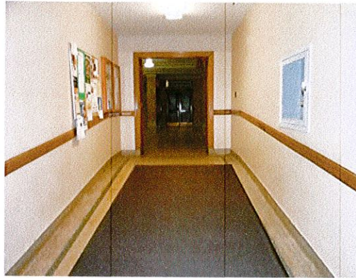
Photo 2: Add handrails along the ramp to the break room (15).
