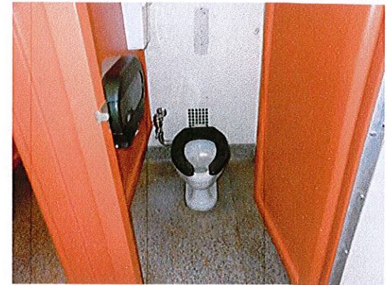
Photo 9: View of typical women's toilet room. Features of accessibility are not provided in the multi-fixture toilet rooms. Post signs directing to the unisex accessible toilet room.
