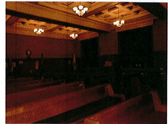
Photo 6: View of council chambers seating area. There is currently 1 wheelchair position. Modify the bench seating to provide additional wheelchair positions (that do not obstruct egress routes).
