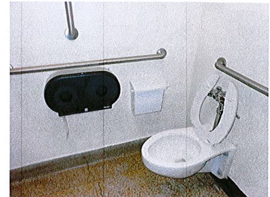
Photo 12: An accessible single user toilet room has been created on 3rd floor. This is a good example of accessibility.
