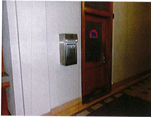
Photo 7: Relocate and lower the pay box on ground floor. It is currently a protruding hazard and the pay slot is located above the reach range.
