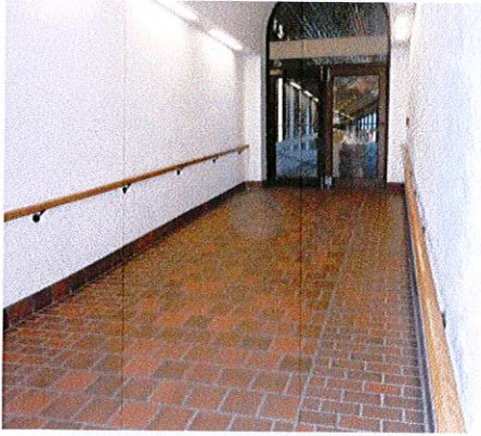
Photo 1: View of skyway entry. There is not a level floor surface for the maneuvering clearance at the doors.
