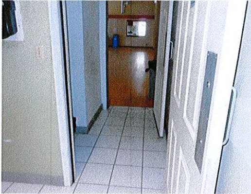
Photo 7: Maneuvering clearance is not currently provided at the entry doors to the upper level toilet rooms.
