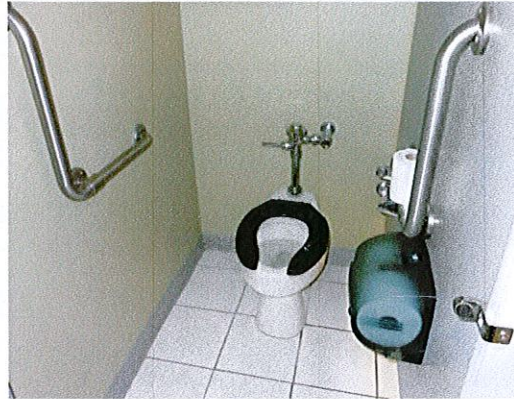
Photo 8: The upper level toilet rooms have been remodeled to provide an ambulatory accessible stall. There is not currently a 60" wide stall.
