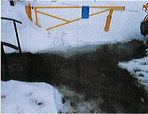
Photo 1: An accessible parking space has been designated near the building. There is currently slope within the parking space causing water and ice to build up.
