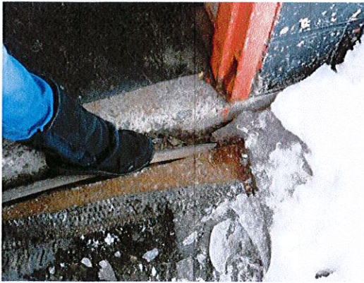
Photo 1: Patch the rise at the main entry.
