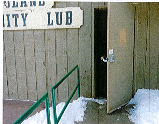
Photo 2: Enlarge the concrete pad to provide maneuvering clearance at the community room entry.
