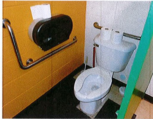
Photo 8: View of lower level toilet room. Currently no features of accessibility are provided.
