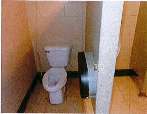
Photo 7: View of existing upper level toilet room. Remodeling is planned to provide features of accessibility.
