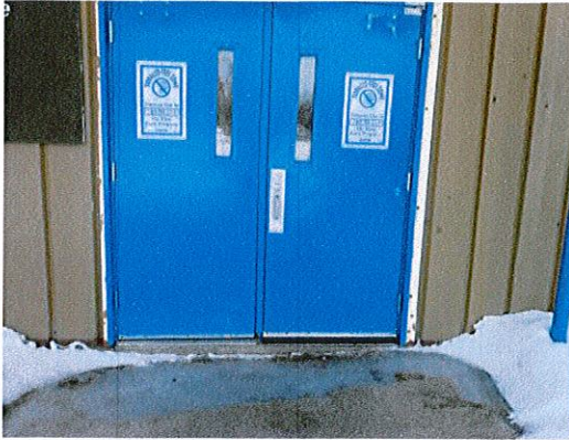
Photo 1: Eliminate the rise at the threshold at the main entry.
