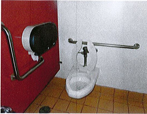
Photo 7: Some features of accessibility have been provided in the upper level toilet rooms of the main building. Replace the "L" shaped grab bar and relocate the toilet paper dispenser to below the grab bar.
