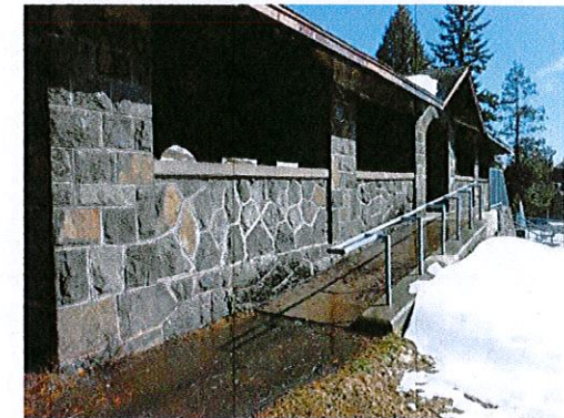
Photo 12: View of picnic pavilion. Add a handrail to the wall side of the ramp.
