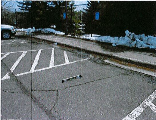
Photo 1: Relocate or modify the accessible parking so the slope does not exceed 2% (currently 6.5%).
