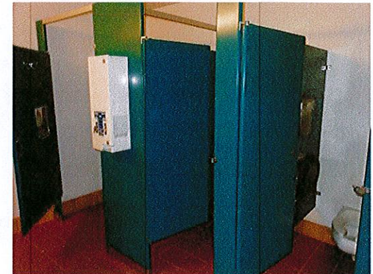
Photo 6: Relocate the product dispenser so it does not create a protruding hazard in the upper level women's toilet room.
