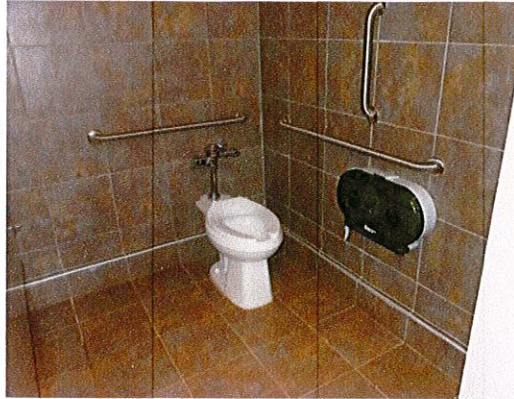
Photo 8: View of lower level toilet in the main building. This is a good example of accessibility.
