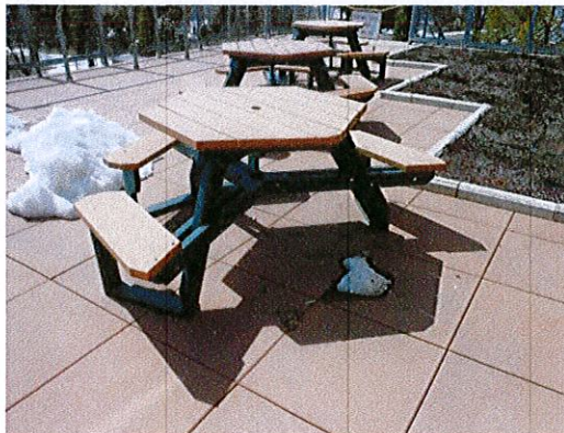
Photo 5: Tables on the deck currently provide positions with knee and toe clearance. This is a good example of accessibility.
