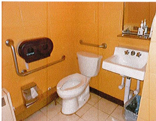
Photo 11: View of single user toilet room in Primate / Nocturnal building. This location is not currently accessible.
