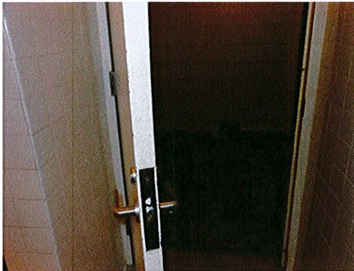
Photo 10: Maneuvering clearance is not currently provided on the pull (interior) side of the toilet rooms in the lower level.
