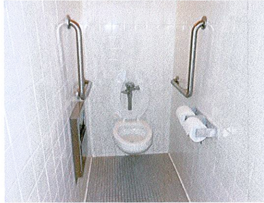
Photo 8: View of typical toilet room. Ambulatory accessible stalls are provided, but there is not a 60" wide accessible stall in the building.
