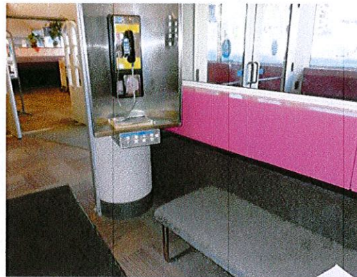
Photo 5: Relocate the bench so it does not obstruct the approach to the pay phone. Lower the phone so the coin slot is 48" max AFF (currently 60").
