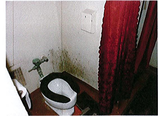
Photo 6: View of women's toilet room. There are currently no features of accessibility provided.
