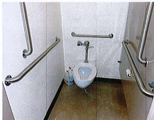
Photo 5: The upper level toilet rooms provide an ambulatory accessible stall, but not a 5' accessible stall.
