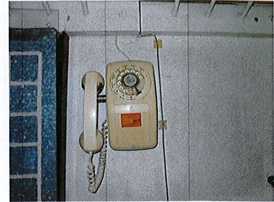
Photo 3: Replace the rotary style phone with a push button style.
