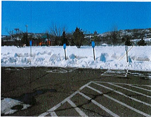
Photo 1: View of accessible parking. Re-stripe to provide an 8' wide access aisle. (Can be shared between 2 spaces.)
