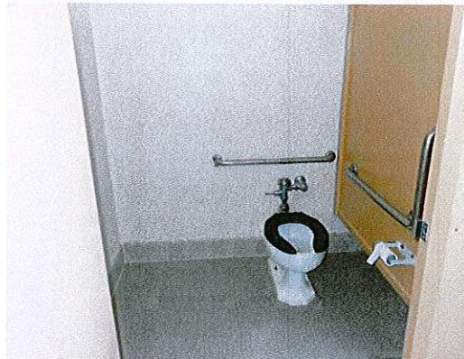
Photo 5: View of men's toilet room. Remodeling has occurred to provide features of accessibility.
