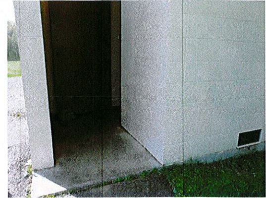
Photo 3: Eliminate the rise at the concrete stoop at the toilet room entry.
