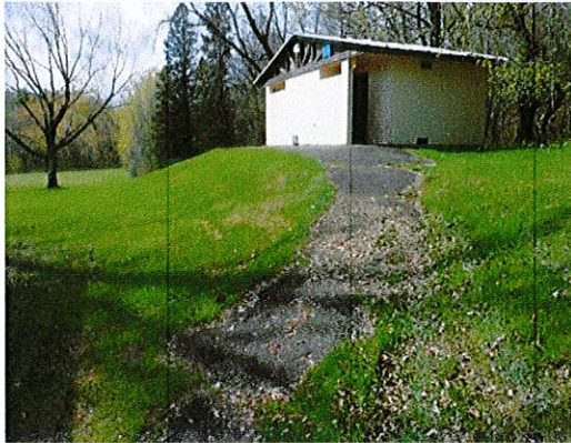
Photo 2: The slope of the route from the picnic pavilion to the toilet room is currently 19.8%.
