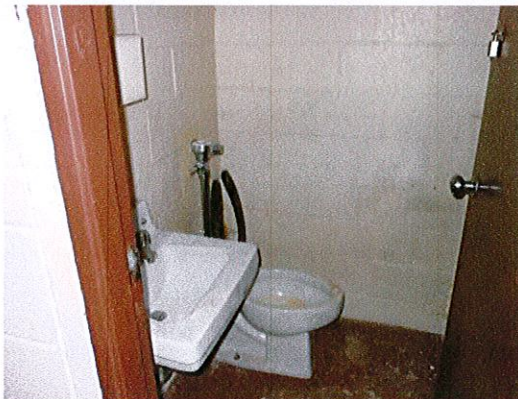
Photo 4: View of lower level toilet room. The toilet room currently provides no features of accessibility.
