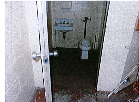
Photo 3: View of upper level toilet room. The toilet room currently provides no features of accessibility.
