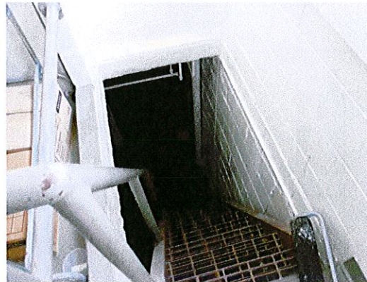
Photo 2: There is not currently an accessible route between levels.
