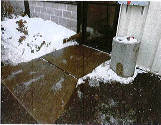
Photo 1: Enlarge the concrete pad to provide maneuvering clearance at the main entry.
