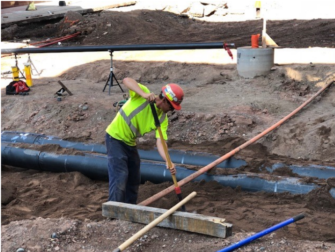
Crews beginning to fill around hot water parts on 4th Avenue W.
